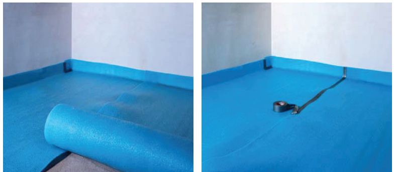
A single layer can also be put side by side (edge to edge) with no overlap. Then a very careful taping with a strong adhesive tape is needed to avoid any screed mass penetration.
